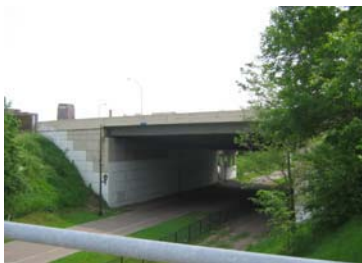
There are 44 bridges that cross the Greenway throughout the length of the project area.
