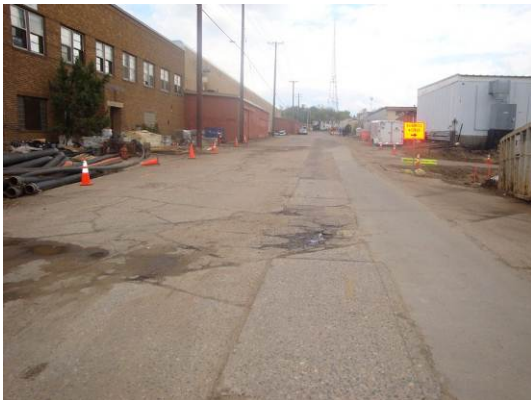
4 th Street SE is in need of reconstruction
