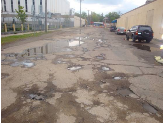
30 th Avenue SE needs to be reconstructed
