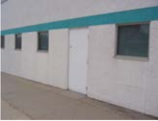
Large, blank wall surfaces should be avoided. Windows, doorways, awnings and other means of articulating facades are encouraged
