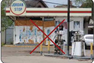
The images above show existing buildings on Lake Street. These parcels should be redeveloped to their highest and best use.
