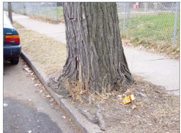
Narrow boulevards can cause damage to sidewalks and inhibit tree health. Photo: An existing boulevard near 31st Street and Chicago Avenue.
